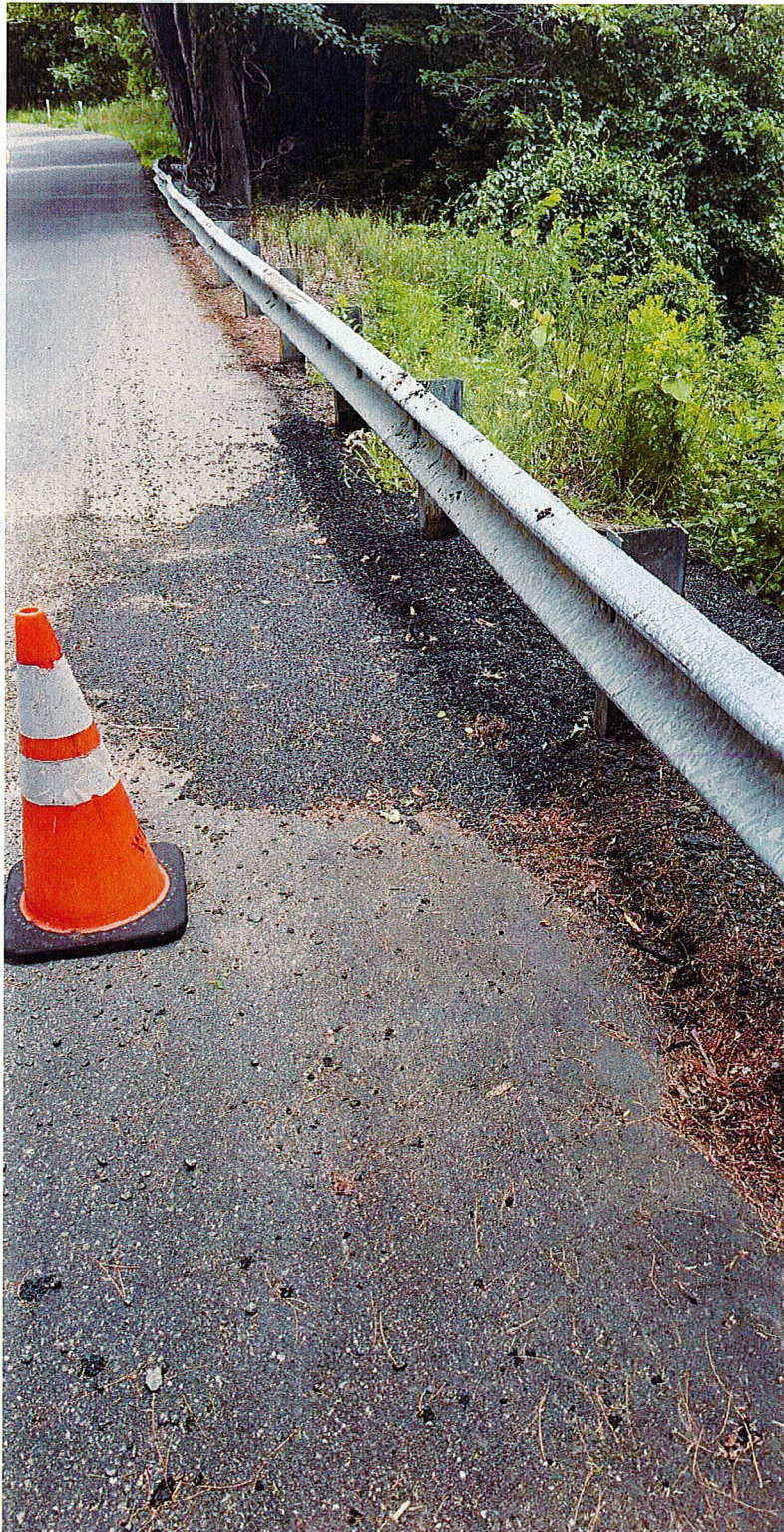
Figure 1 Patched sinkhole on East side of road. Photo taken facing North.
